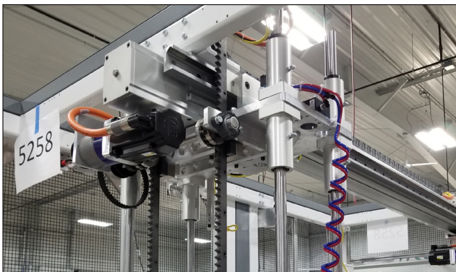
In the food product packaging industry, a LoPro system provides long overhead actuation for an automated material transfer system.
